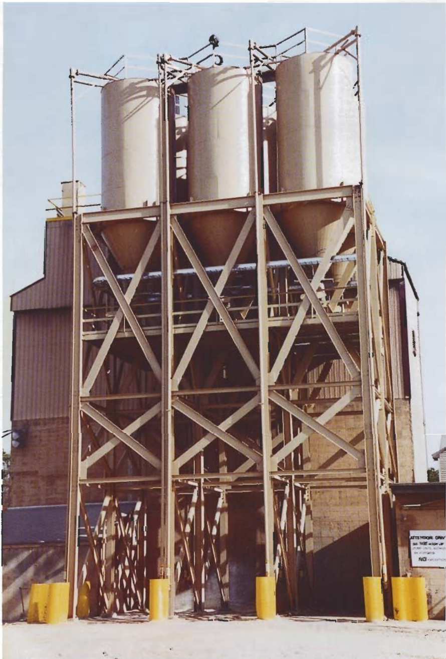
The new 100-ton-capacity silos are installed outside the production facility approximately 80 feet above the ground.
